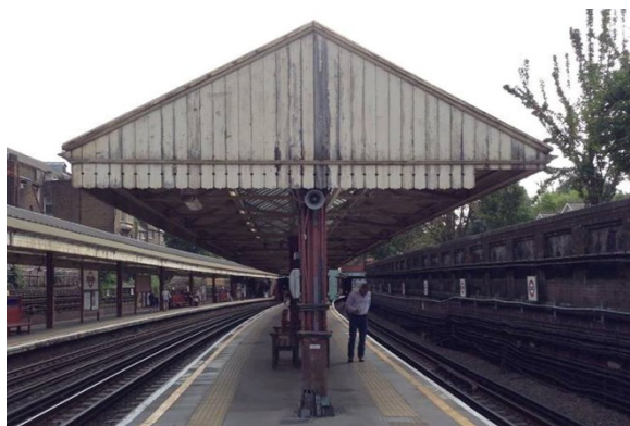
Figure 14. Barons Court stations' train-sheds with steel column and timber panels as coverings (Fieldwork, 2016).
