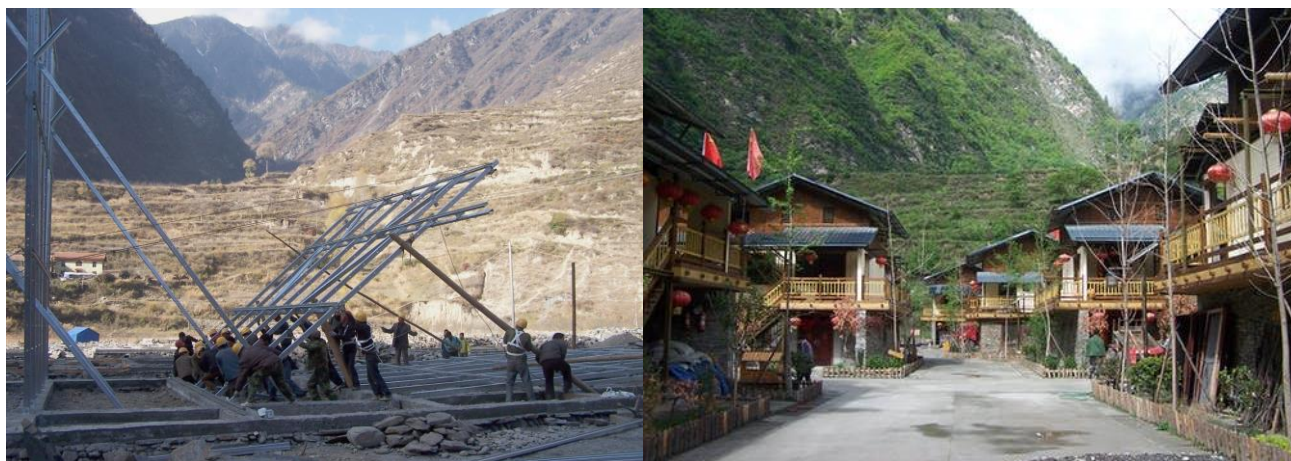
Figure 3. (Left) Qiang people erect the light-steel frames of their houses; (Right) The street view of the village (Architect.com, 2012).
