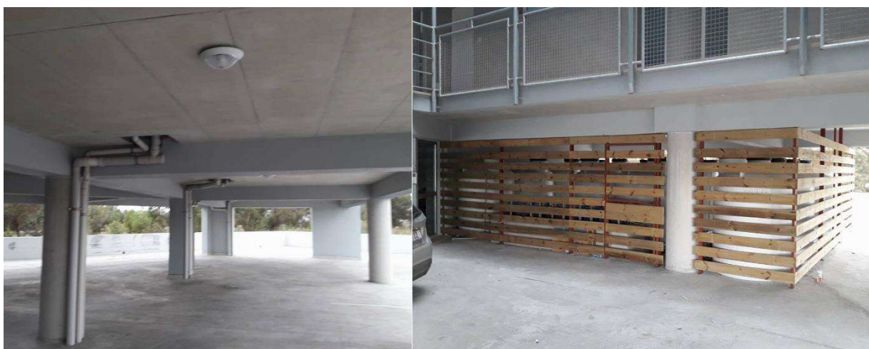
Figure 14, (River Side Residential Hostel Water Tanks and System) (URL 14)
