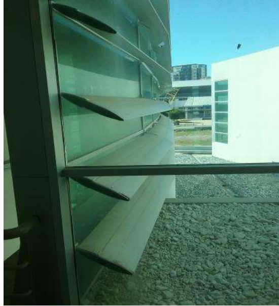
Fig 9. Continuous Horizontal Aluminium Fins Employed on Upper Facade of Lemar Building (Chinweokwu and Alibaba's Archive, 2017)
