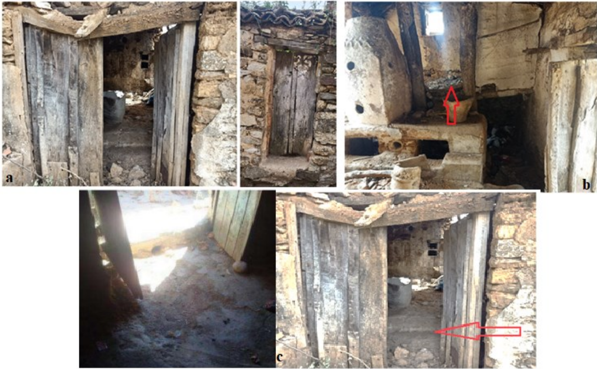
Fig 6: House elements a- main door. b- Small room below the stable. c- The Threshold
