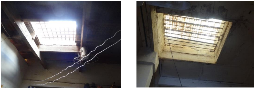
Fig 6. Pictures showing the rozna on the roof in the wasr eddar of H T11 , H T15 .
