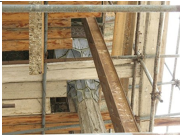
Using beams to support the weight of the roof in the absence of column load-bearing capacity.
