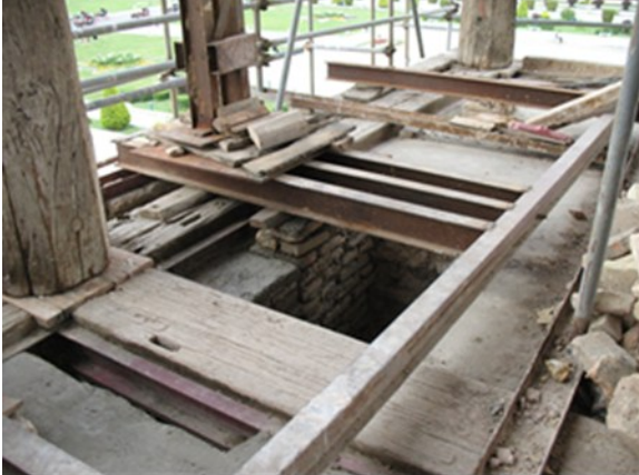
Installing iron beams on the floor and the column itself, and using wooden crossbars on the iron beams and at the base of the column in Aalighapu.
