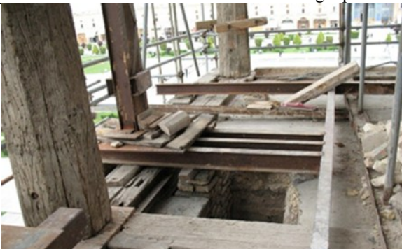
Installing the column timbers using special wood adhesives on both sides of the columns to hold the two pieces of column timber together.
