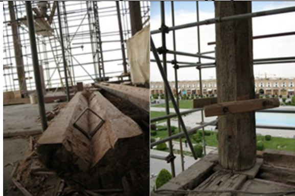
(Left) Cutting the column timbers in half to fit the iron beams inside them. (Right) Wood is placed on both sides of the column to hold the two parts of the column together.
