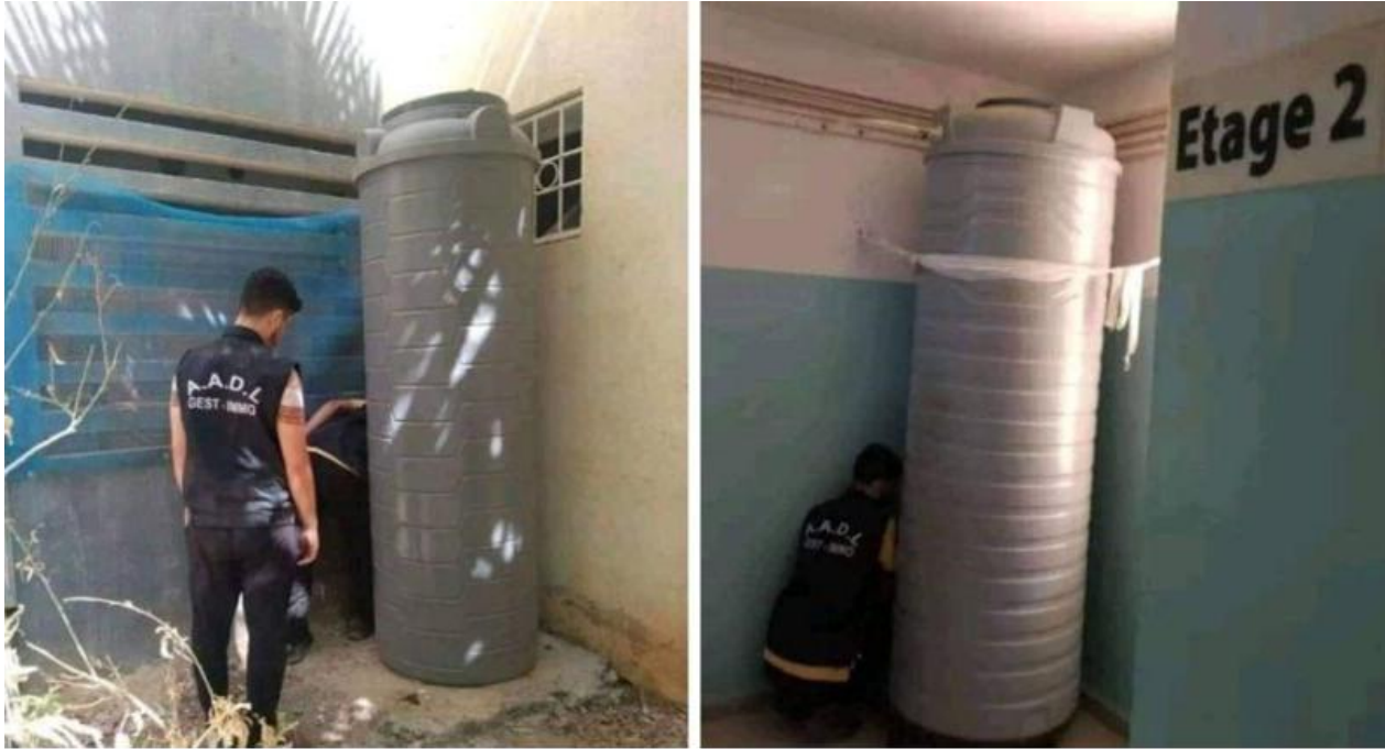
Figure 3. improvised water reservoirs installed within shared spaces in the AADL housing program (Developed by the Authors).
