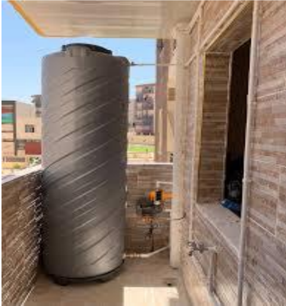
Figure 5. The tanks Placed on balconies (Developed by the Authors).
